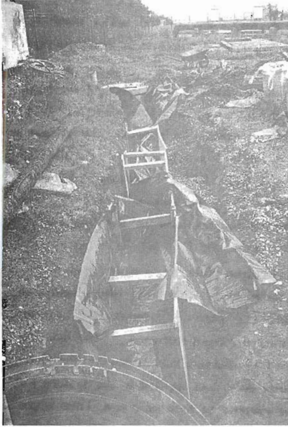
Plate (1) the filter is excavated and lined with an impermeable geotextile warp
