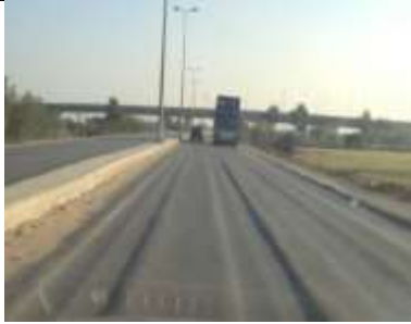
Figure 2. High Severity Rutting (Mansoura-Gamsa Road)
