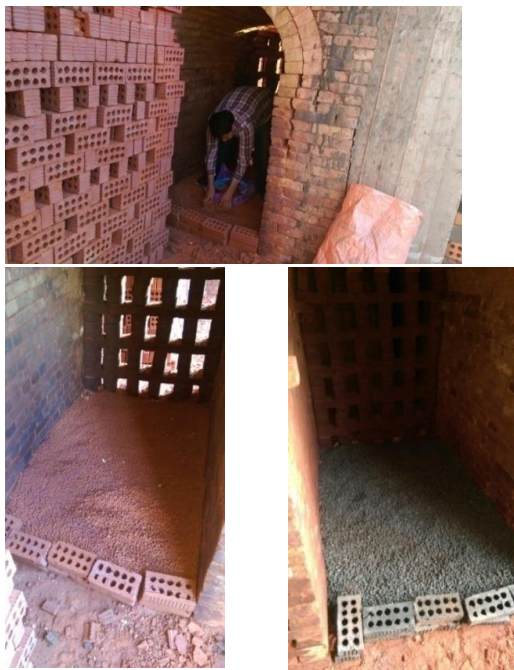
Figure (3): Firing up to 1000 °C in brick factory in Nawsa village- Mansoura –Egypt
