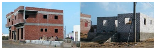
Fig. 9. Photos showing construction problems in the Graduate Villages project site (10).
