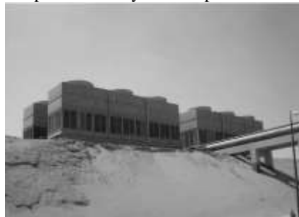
Fig. 15. Cooling towers at AUC's central utility plant.[36]
