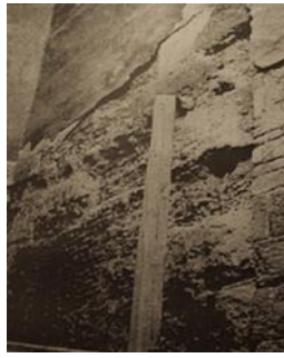
Fig (2) stone and masonry failure caused by the gypsum plastering used for restoring the wall of Qawsun gate (JERE L1995)
