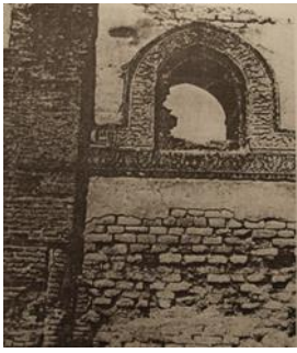
Fig (1) the deterioration of the northern wall of al- Azhar mosque due to the humidity and the wind factors in 1915 (JERE L1995)
