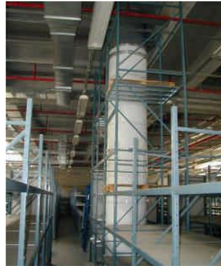
Duct Unit (D=90 cm, L=13m)
